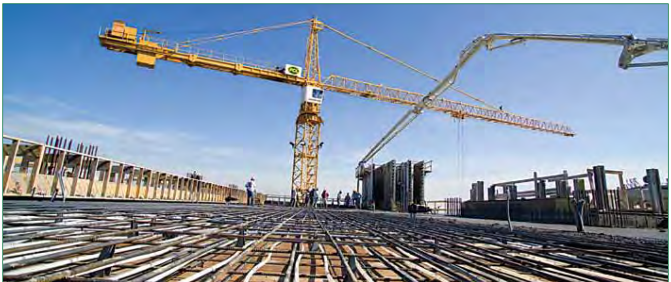
Construction takes place on a variety of fronts in April, July, August and October 2007
