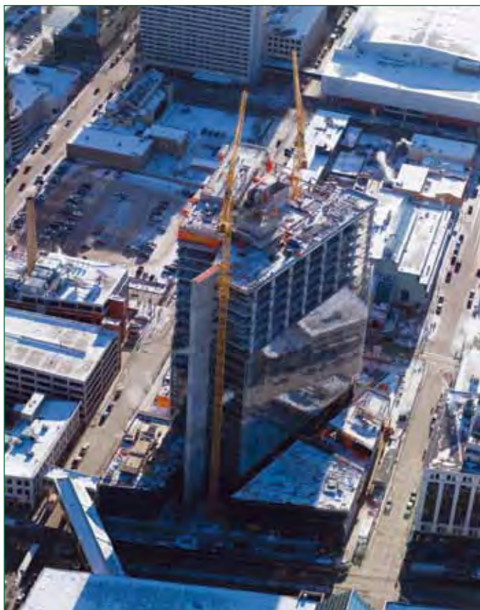
An aerial view of the new downtown office revealing its dramatic design and shape.
