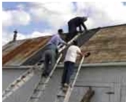
The 'work gang' installs a membrane on the roof. From top: Georges Jobin (consultant builder), Pierre Huberdeau, 'Foreman' Raymond Theroux and John Quayle.
