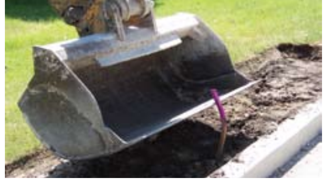
Survey monument destruction
