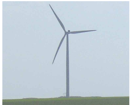
Wind energy projects will move forward in 2007-08.
